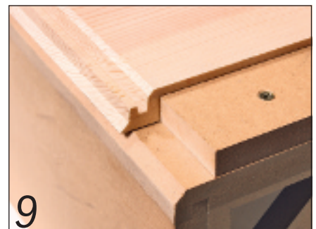
9 The finished cut reveals the very large glue area which gives the joint its strength
